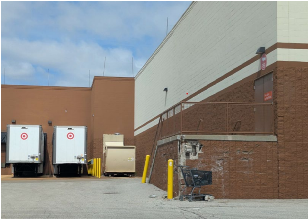
Ex.5b at P_12066 (damaged bricks at nearby Target).
