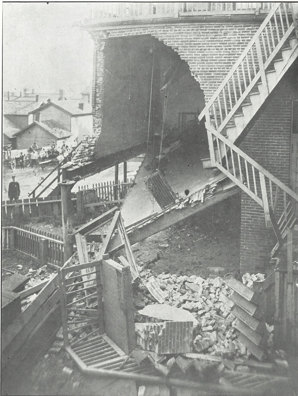
The World Theatre, Scranton, Pa., wrecked by a mine cave shortly after the audience had been dismissed for the night. Had this occurred shortly before the time of the collapse of the building, hundreds of lives would have been sacrificed to the greed of mining operators, now seeking to avoid remedial mine cave legislation.
